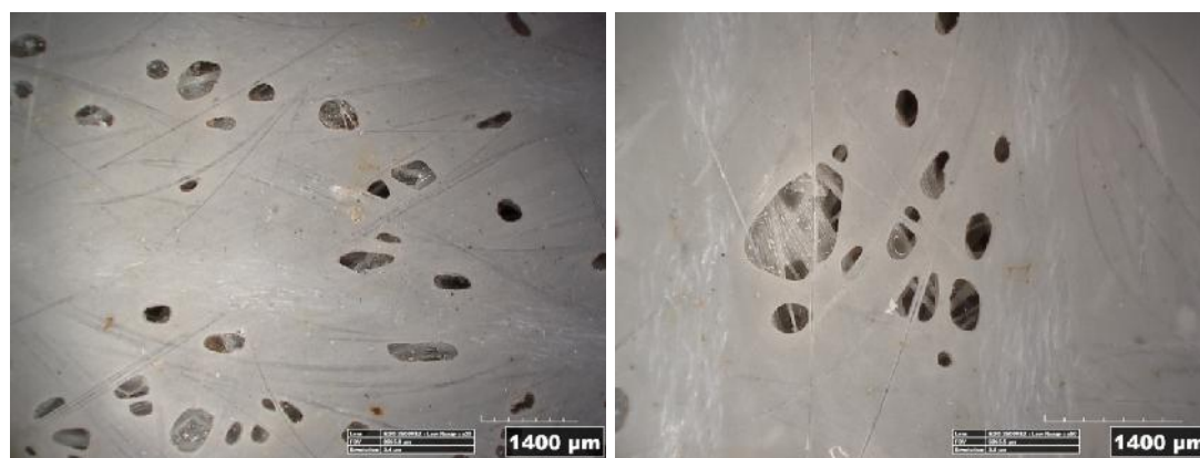
Fig. H-35. Existing voids in unconditioned specimens' exterior surface
